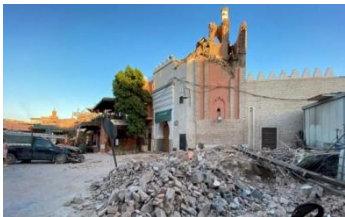
A view shows damage at an old mosque in the historic city of Marrakech, following a powerful earthquake in Morocco, September 9, 2023 [https://edition.cnn.com/2023/09/10/africa/mosque-earthquake-damage-marrakech-intl/index.html]
