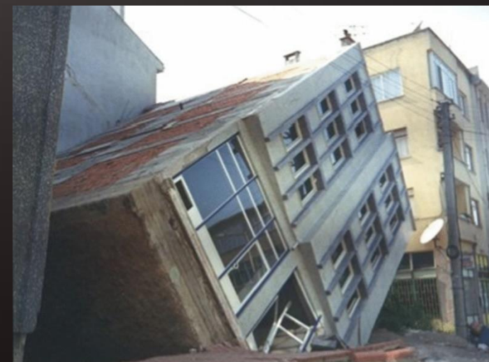
Example of an overall rotation of the base of the structure with an overturning motion during 1999 Kocaeli earthquake, Turkey [Bozzoni, F. et al., Bull. Earthq. Eng. 2021, 19, 4719–4744]
