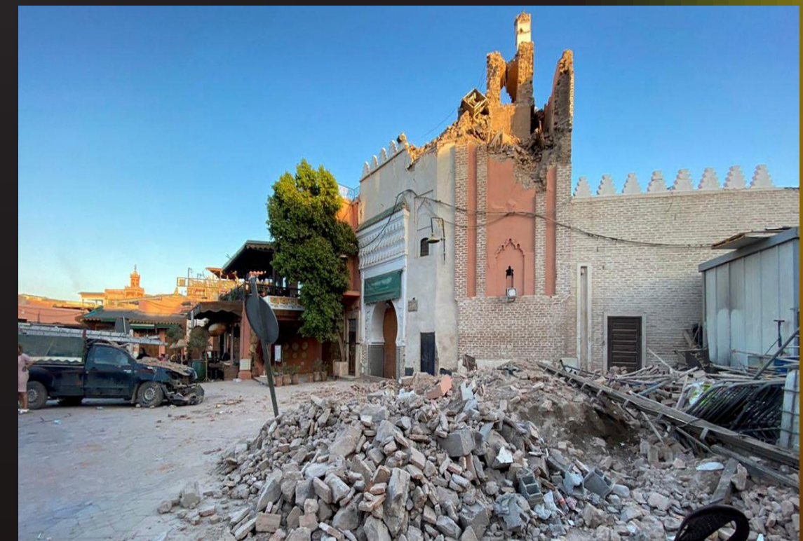
A view shows damage at an old mosque in the historic city of Marrakech, following a powerful earthquake in Morocco, September 9, 2023 [ https://edition.cnn.com/2023/09/10/africa/mosque-earthquake-damage-marrakech-intl/index.html ]
