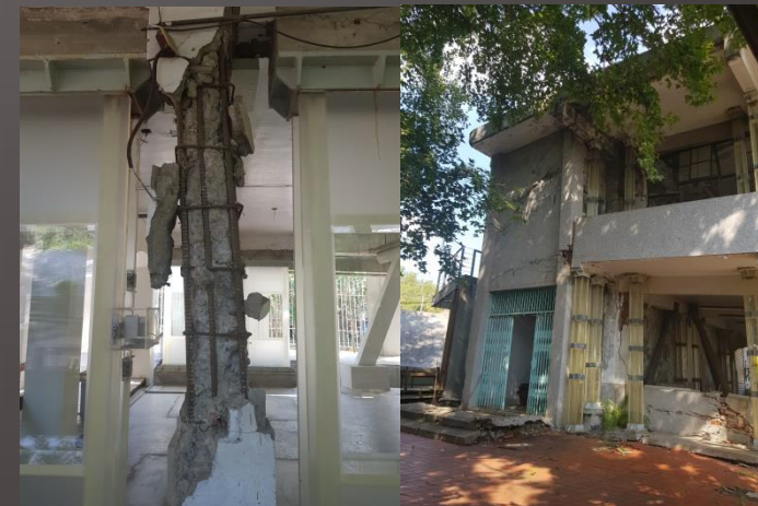
Damages in building after September 21, 1999, a strong earthquake of 7.3 in the central part of Taiwan, presented in 921 Earthquake Museum of Taiwan
